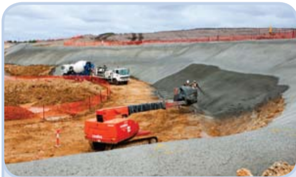
Plant site: The box cut is sprayed with concrete – a process known as 'shotcreting'
