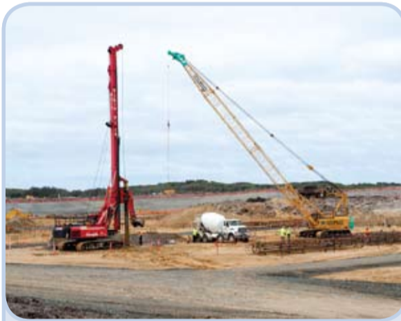
A piling rig and crane at work installing concrete piles, which provide support for the pre-treatment structures.
